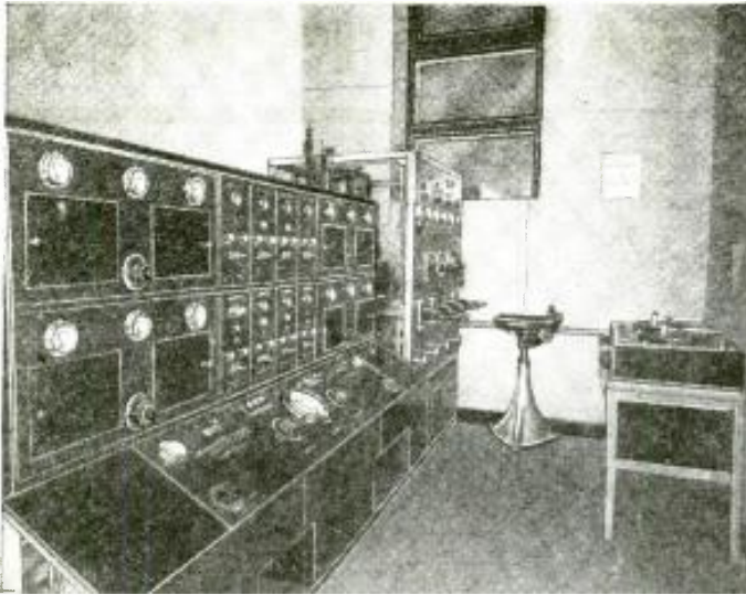
The "technical room" at the 150 kw. Luxembourg station.
